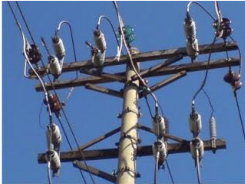
Gambar 7. Disconnecting Switch (DS)
