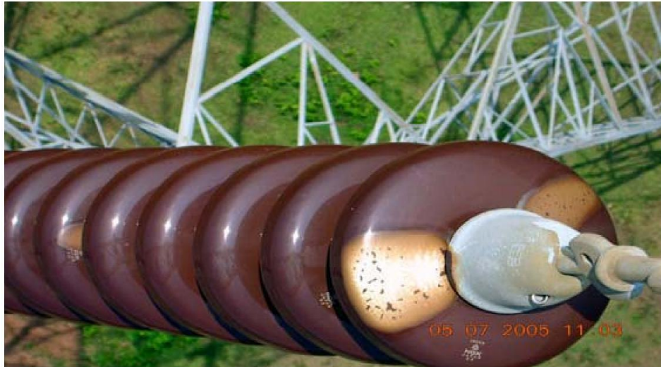
Gambar 9.2 Kerusakan (abnormality peralatan).pada Isolator
