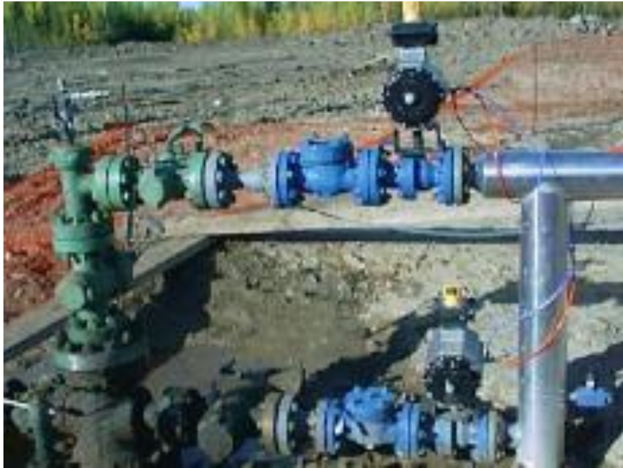
Gambar 7 Kepala Sumur (Well Head)
