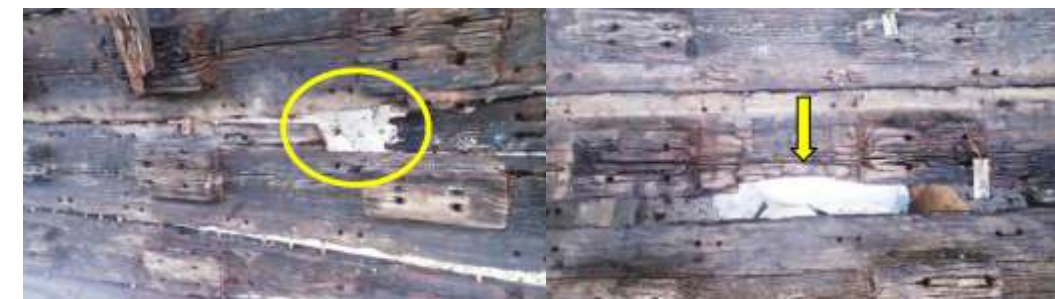
Figure 14. Damaged Planks Caused by a Flaking Process. (Source: A. Mochtar, 2 January 2018)
