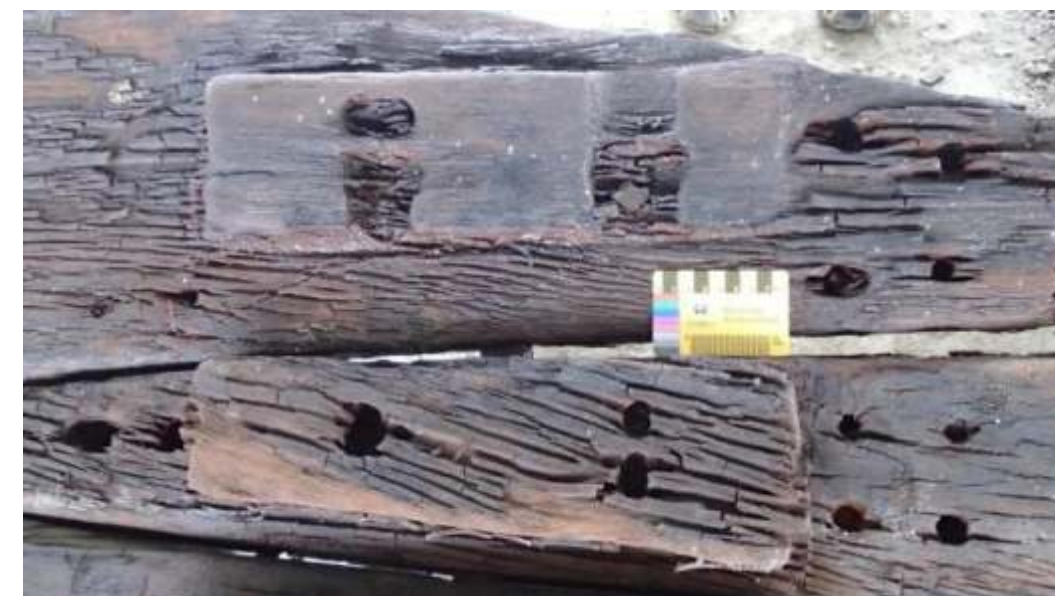
Figure 15. Deformation of a Lug (upper), After Long Exposure to Coastal Weather. (Source: A. Mochtar, 29 December 2017)
