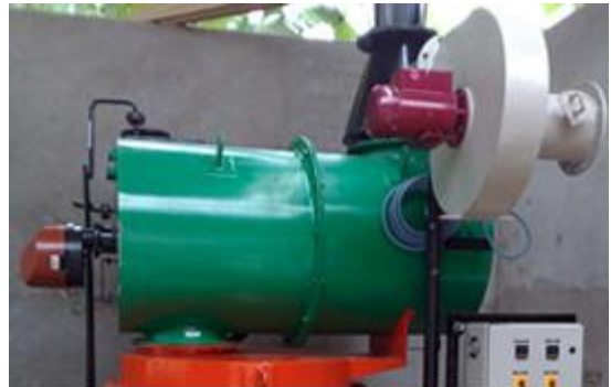
Secondary Combustion Chamber
